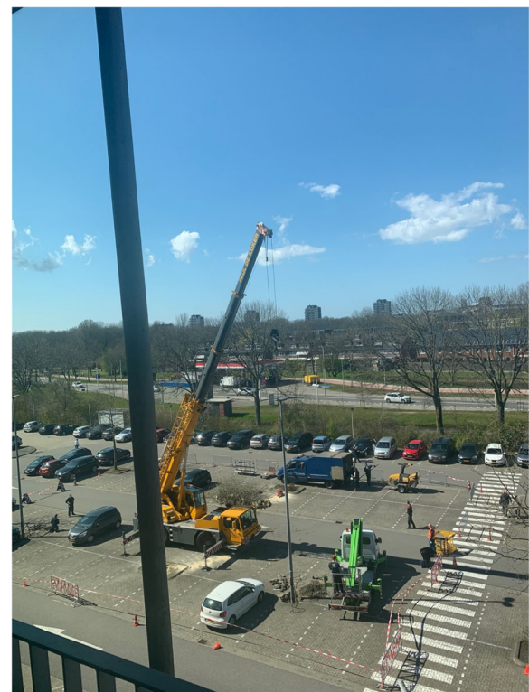
Fig. 1 Construction of an ALS at the parking lot of Alrijne Hospital, Leiderdorp, the Netherlands
